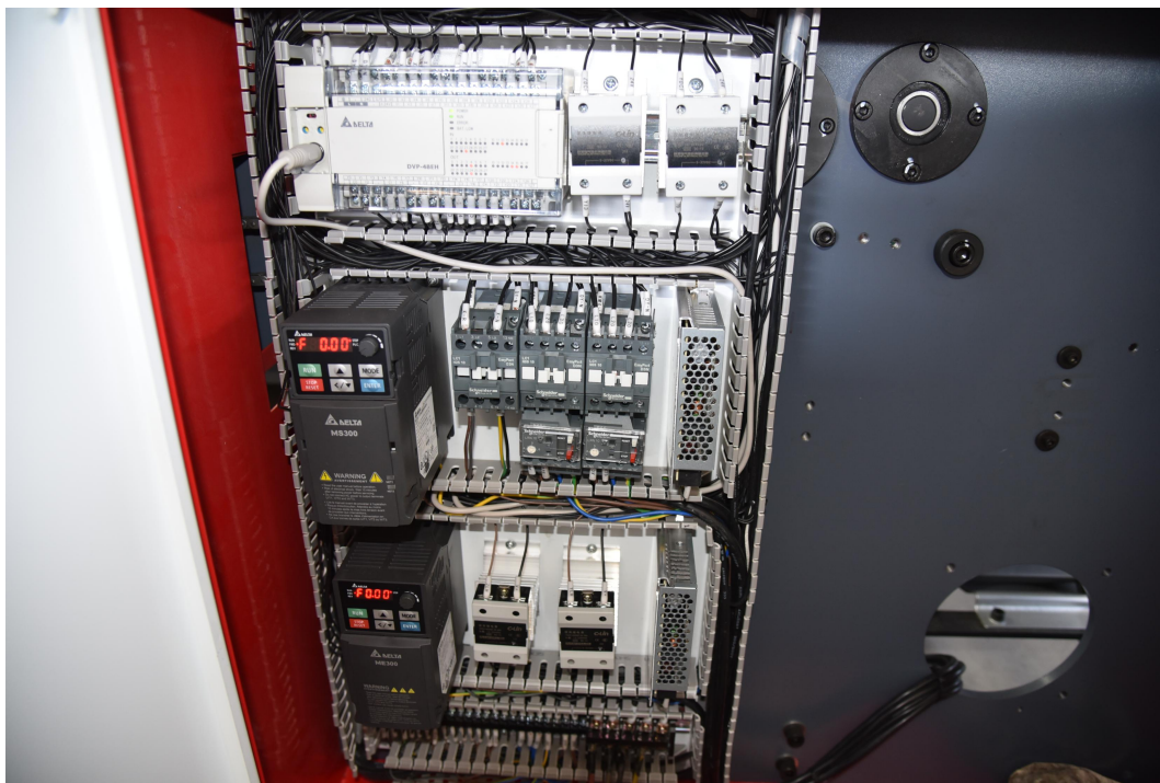
DELTA ELECTRICAL SYSTEM TO KEEP THE MACHINE WORKING STABLE
